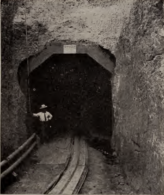
Valley or West Portal of the Gunnison Tunnel, on Line of D. & R. G.
